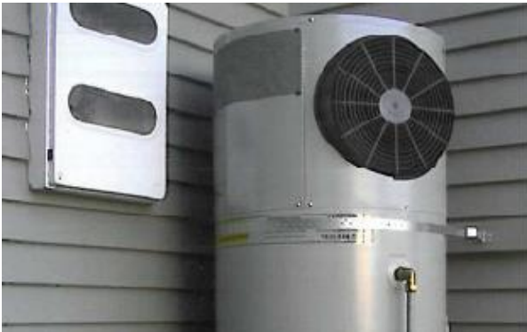
An integral heat pump hot water cylinder is usually sited outside - BRANZ Bulletin 529 Dec 2010
