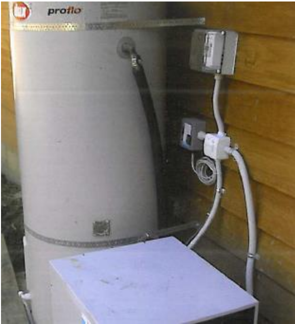
A split heat pump hot water system – the cylinder can be inside the house.
